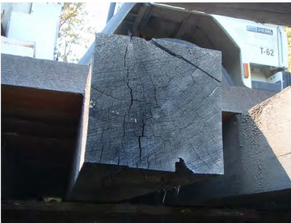
Figure 1-9: Typical condition of ends of deck ties.
