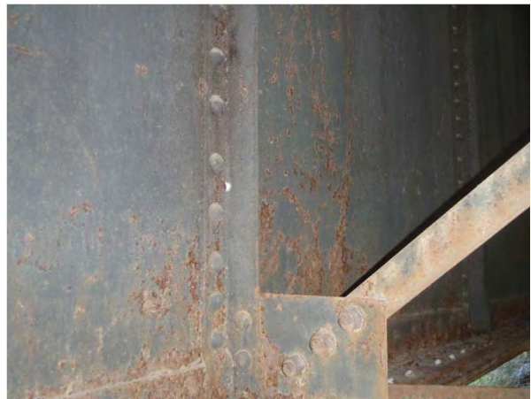
Figure 1-12: Typical condition of steel girders (note minor paint flaking).
