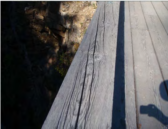
Figure 1-7: Typical wide checks in curb rails.
