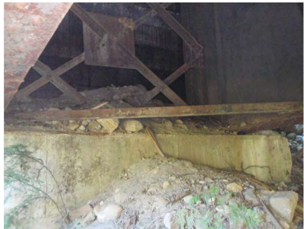
Figure 1-24: Debris at woods end abutment.
