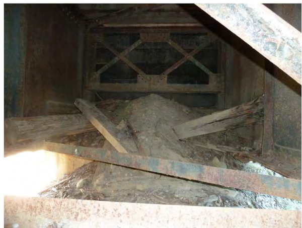
Figure 1-18: Debris at camp end abutment.
